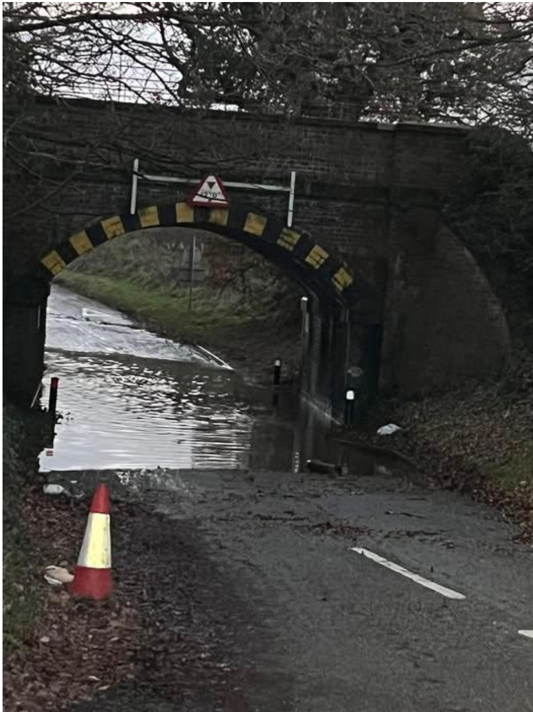
Photograph 4 - Flooded railway underbridge Allscott
